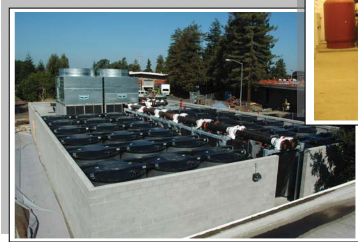
Ice Storage Plant
