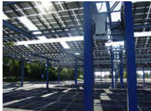
Photovoltaic Panels Covering Parking Lot
